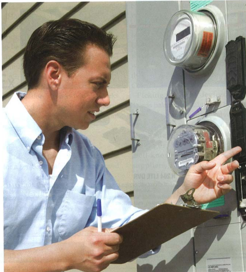
▲ Smart grids can perform automatic meter readings and keep tabs on energy use citywide.
